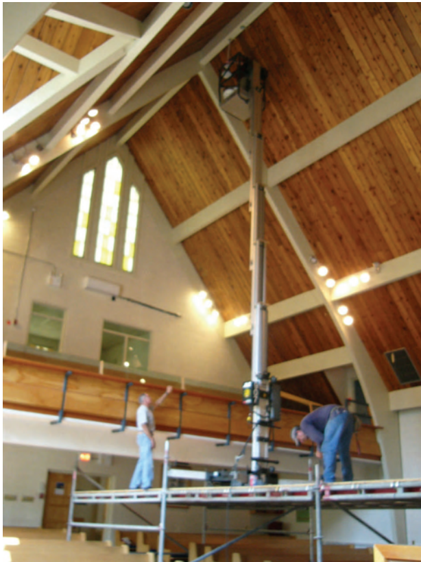
Bob Steed on the left overseeing the installation of new ceiling fans in the sanctuary
